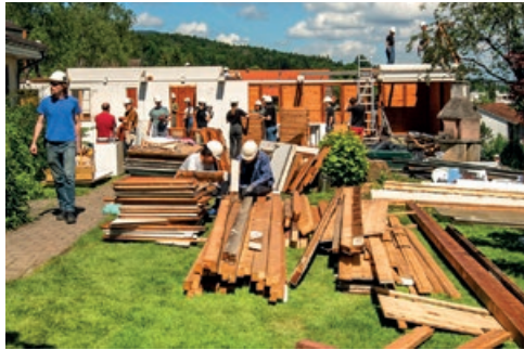
Disassembly of Oetwil am See Music Pavilion for Reuse © Buser Hill Photography, CEA lab
